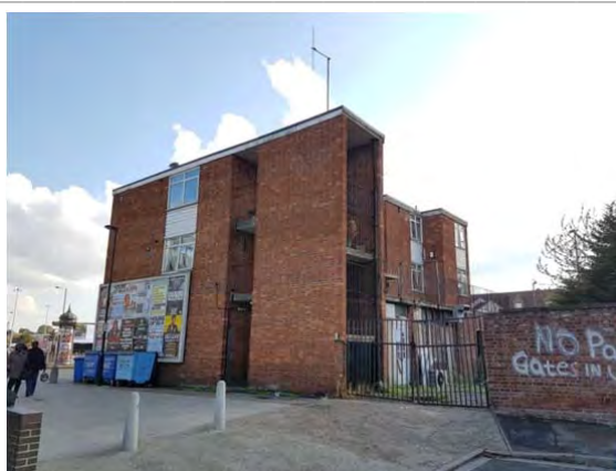
North and West (rear) elevations and access to rear yard from Holmshaw Way
